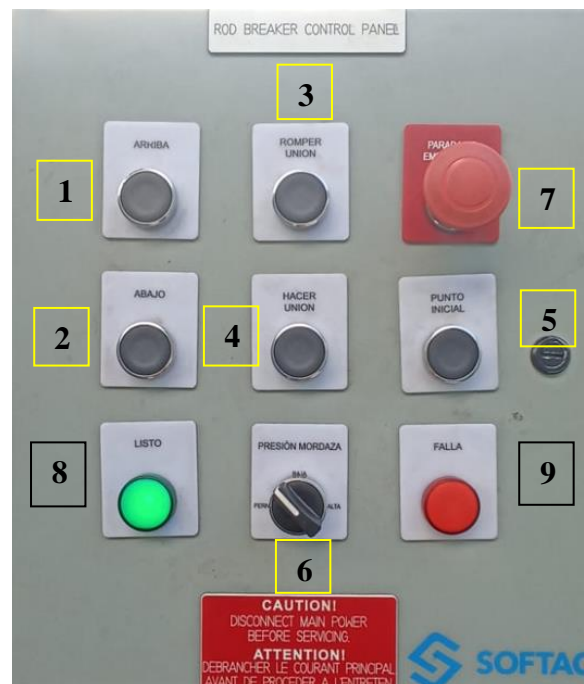
Figura 1. Panel de control rod breaker
